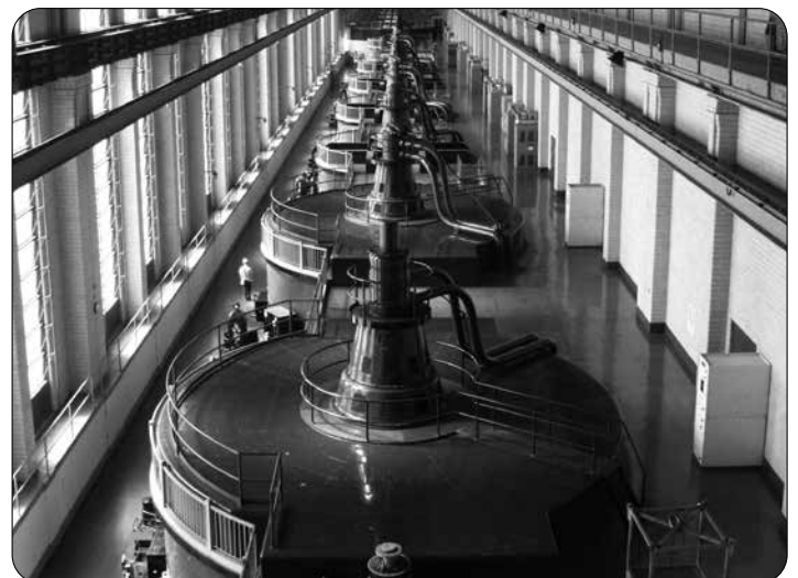
Generators at a hydropower plant.
